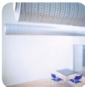
Ventilation duct systems
