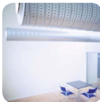
Ventilation duct systems
