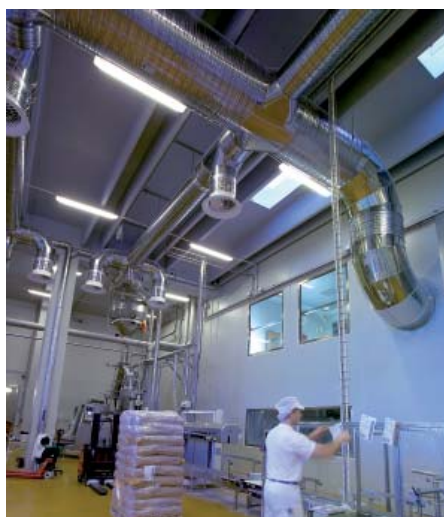
Stainless steel duct system at Arla in Vimmerby in Sweden.
